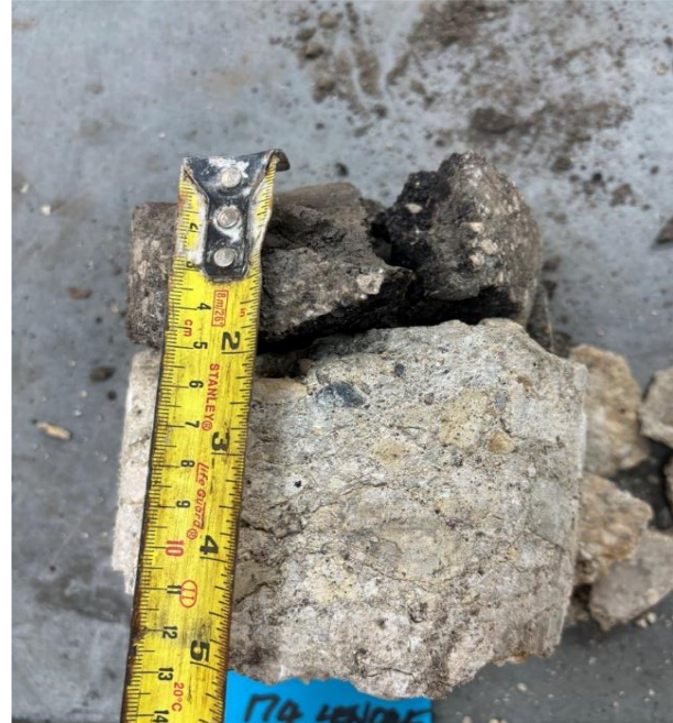
Ruby St - Lenore St Backlane, NBL, Core 38 (Asphalt Thk 51mm; Conc Thk 102)
