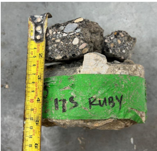
Ruby St - Lenore St Backlane, SBL, Core 39 (Asphalt Thk 40mm; Conc Thk 80)
