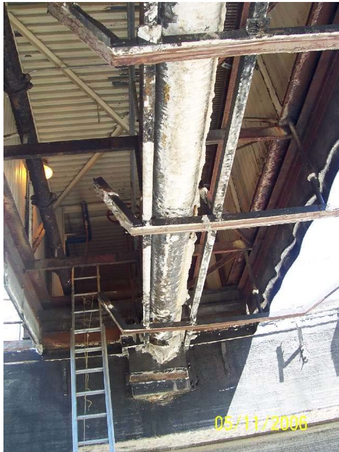
Photo 1-2 Scum Trough & Discharge Box
