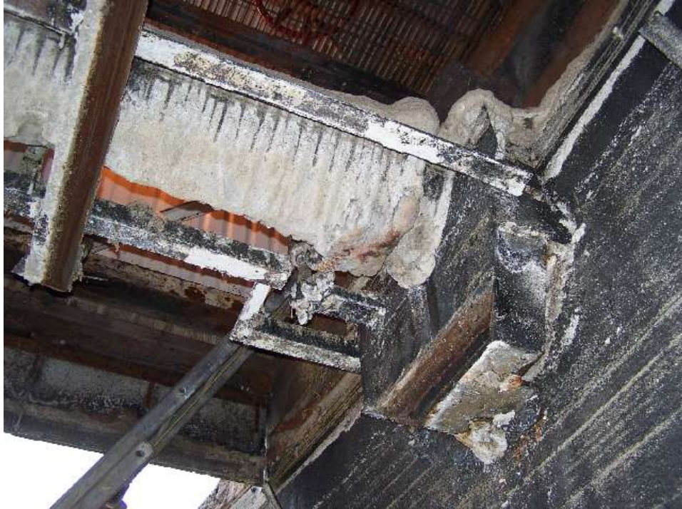
Photo 2-1 Scum Trough Discharge Box
