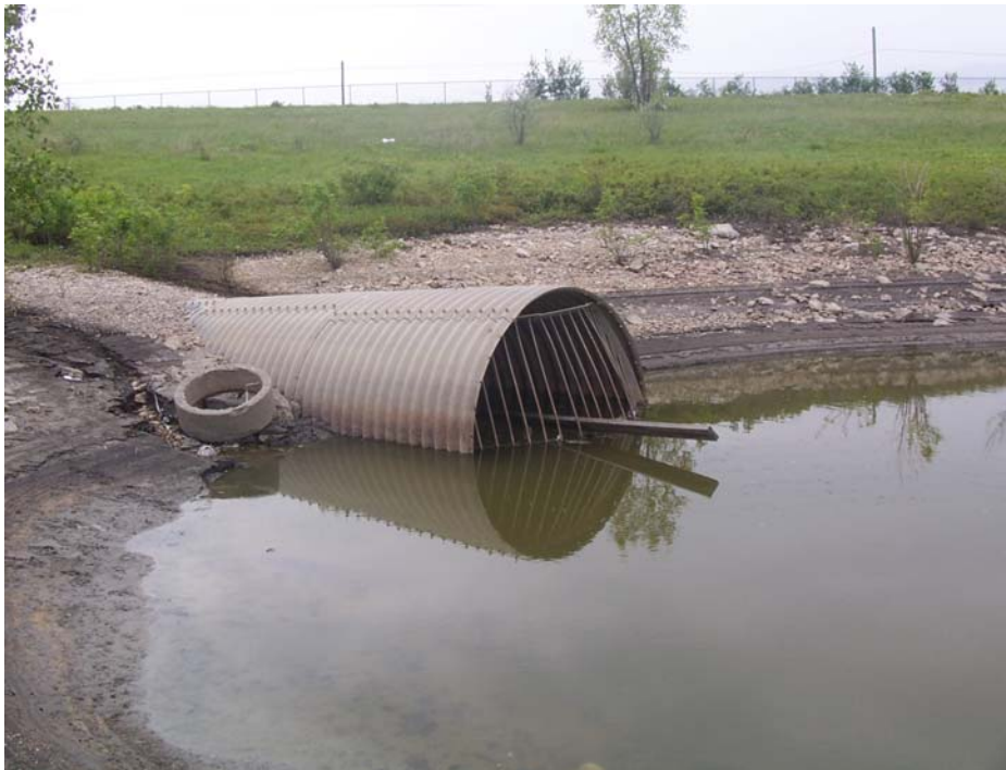
Photo 12 – Intake Pipe (April 10, 2007)
