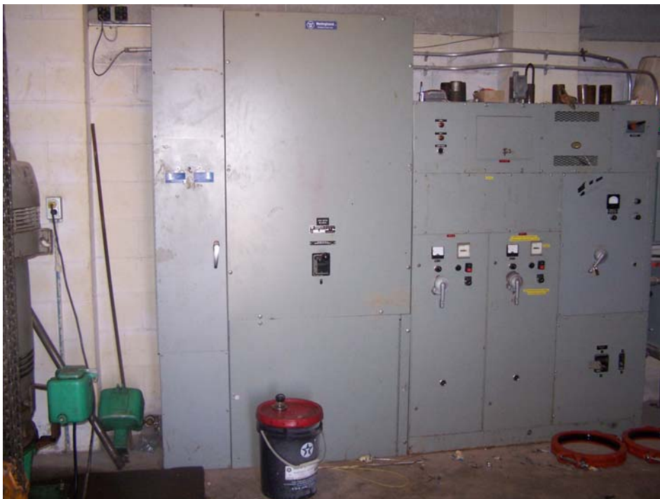
Photo 4 – Existing Pump motors to be removed (main floor)
