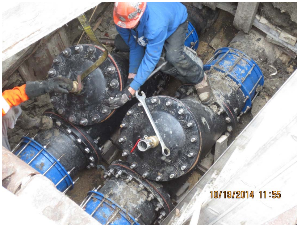
Figure 2 – Existing Tool Launch Wye's Installed Adjacent to Existing Valve Chamber on Assiniboine Crescent.
