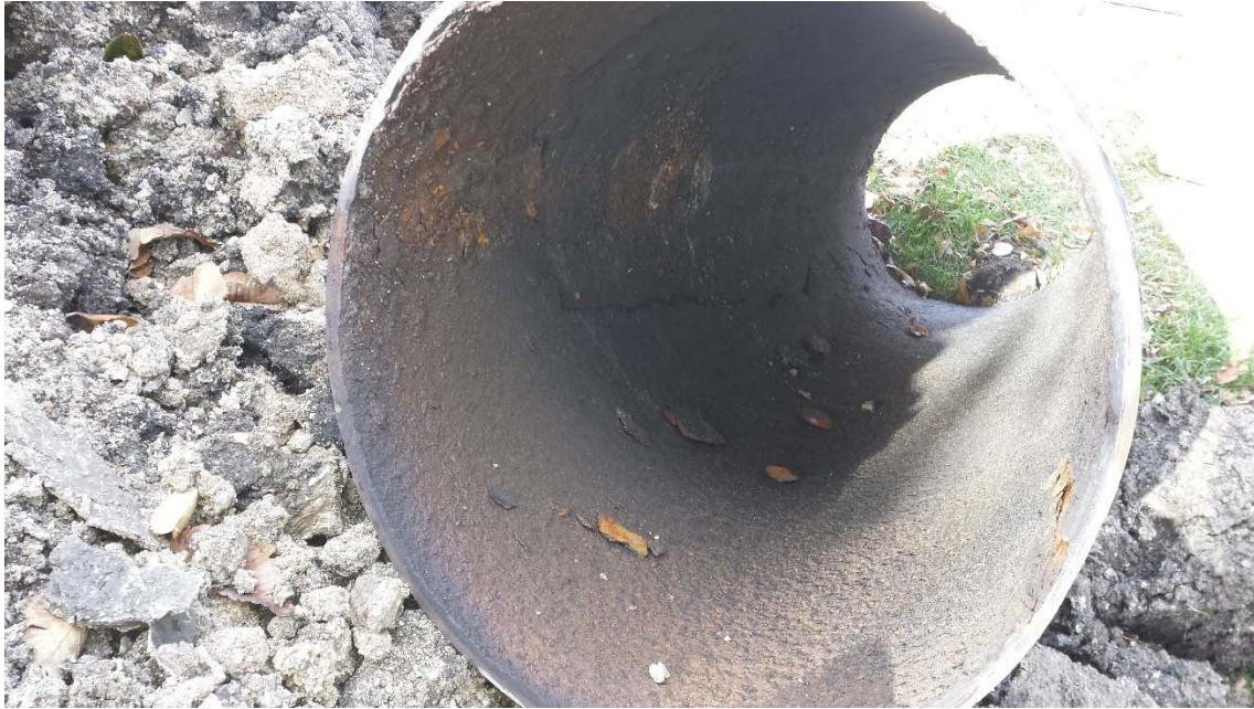
Figure 3 – Interior of St. James Force Interceptor Main Pipe Sample Removed in 2014.
