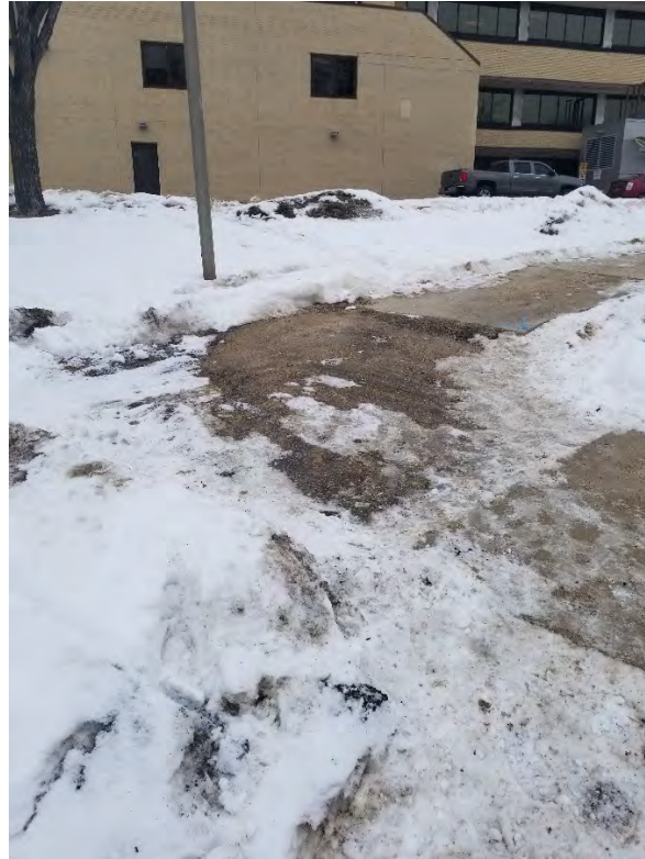
Figure 1 – Existing Sidewalk Repair on North Side of River from Launch Wye Assembly Installation, looking North.
