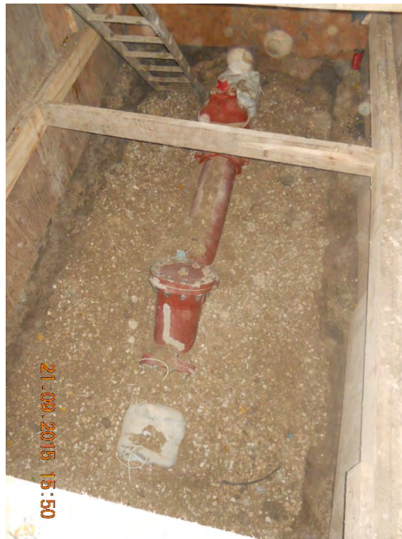
Figure 4 – Existing Launch Wye and Valve Installed on South Side of River.
