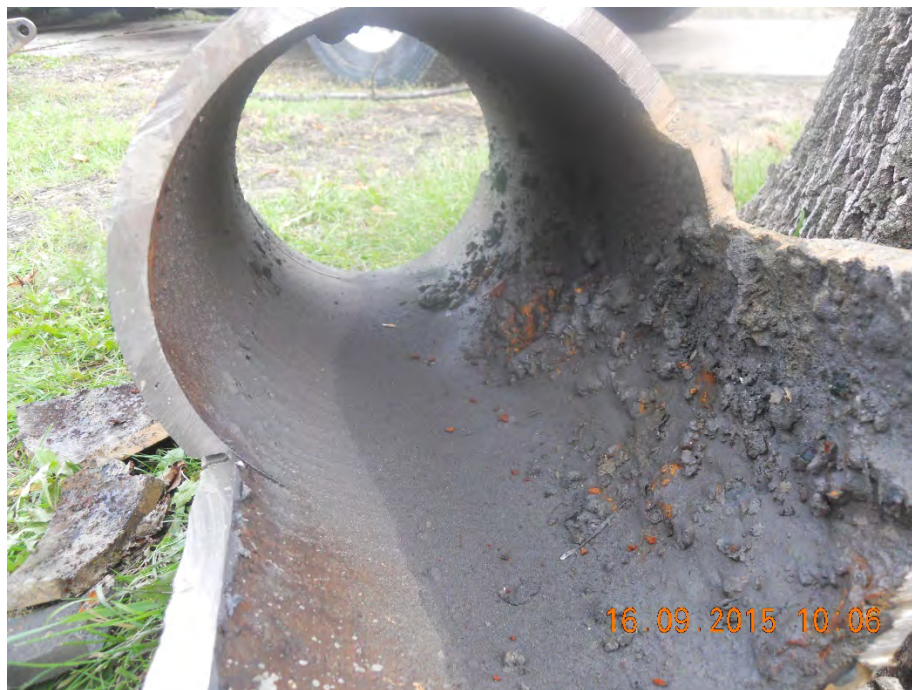
Figure 6 – Cast Iron Water Main Sample Cut during Launch Wye Installation in 2015.
