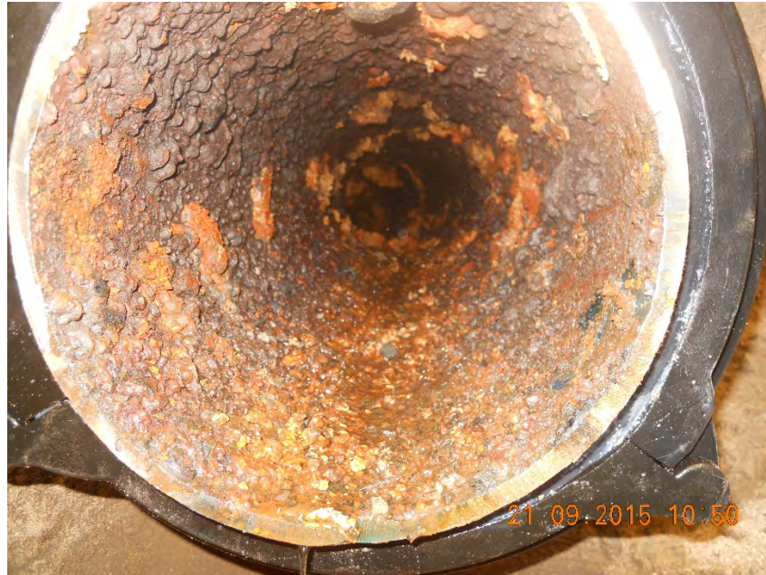
Figure 5 – Steel Water Main Sample Cut during Launch Wye Installation in 2015.
