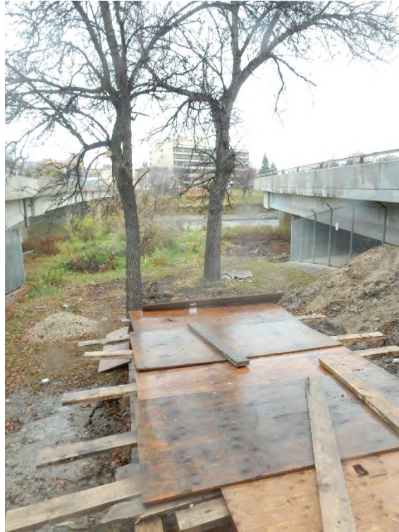
Figure 3 – Excavation location on South Side of River from Launch Wye Assembly Installation, looking North.
