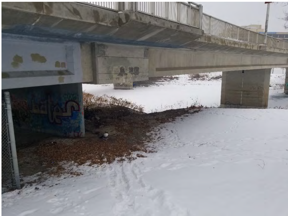
Figure 8 – East Bridge Structure and Access Location to South Side of River, looking Northwest from Access Gate.
