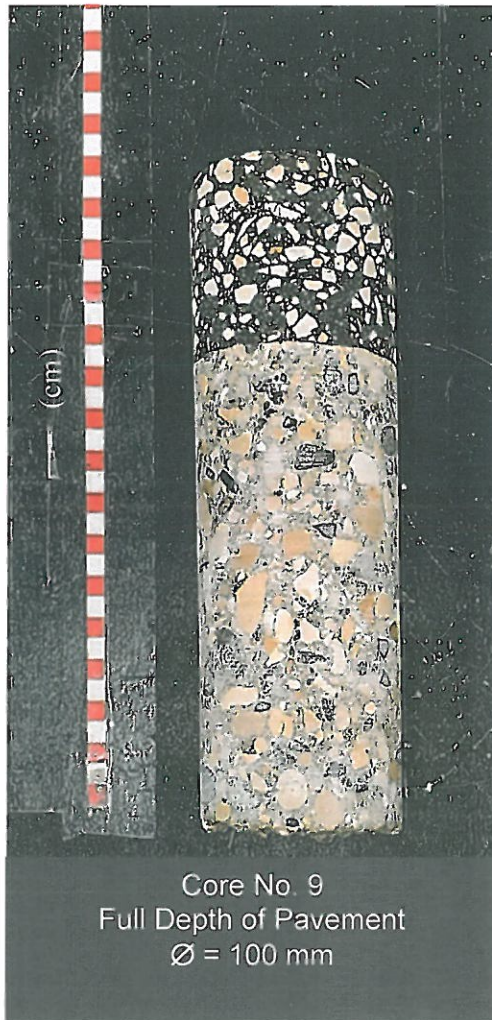
Photograph 29: Intact Specimens from Lagimodiere Boulevard
