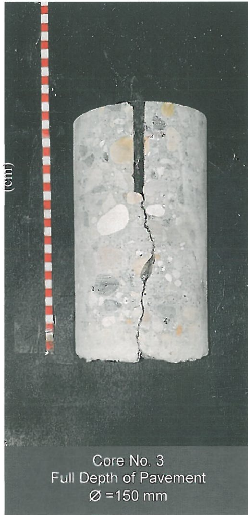
Photograph 3: Intact specimens from Keewatin Street
