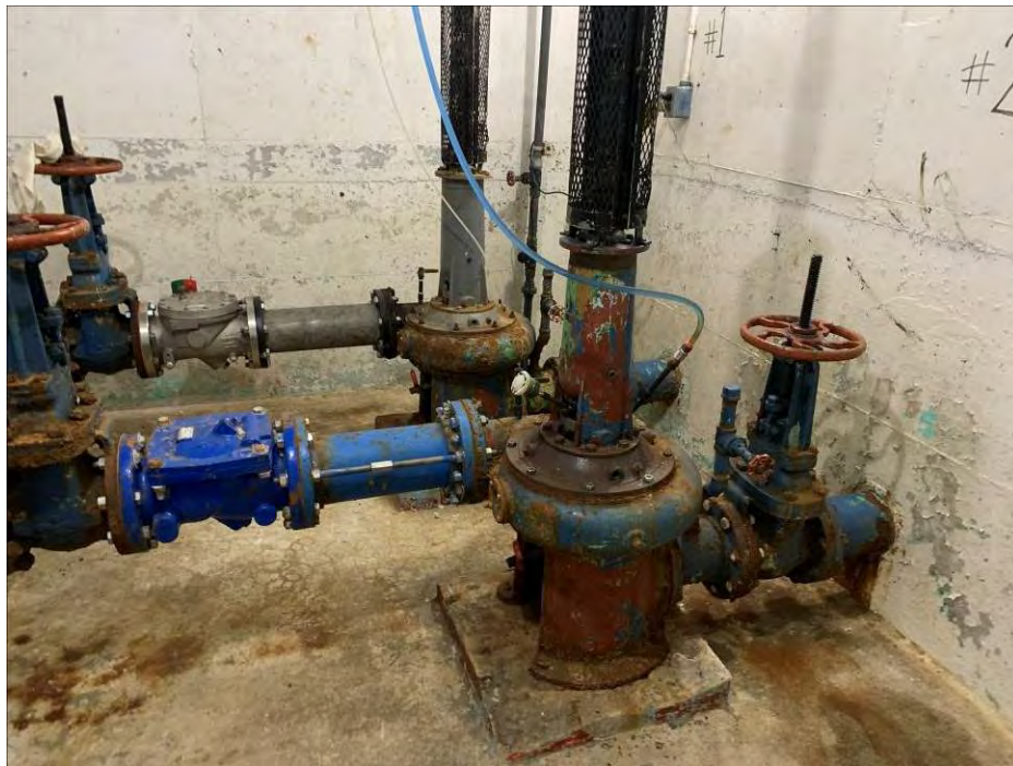
Photo 30: General view of the pumps in the pump chamber. (April 27, 2021)
