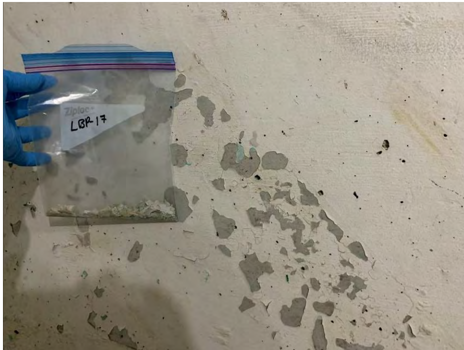
Photo 29: General view of the paint chip sample LBP-17 location on the wall of the pump chamber. (April 27, 2021)
