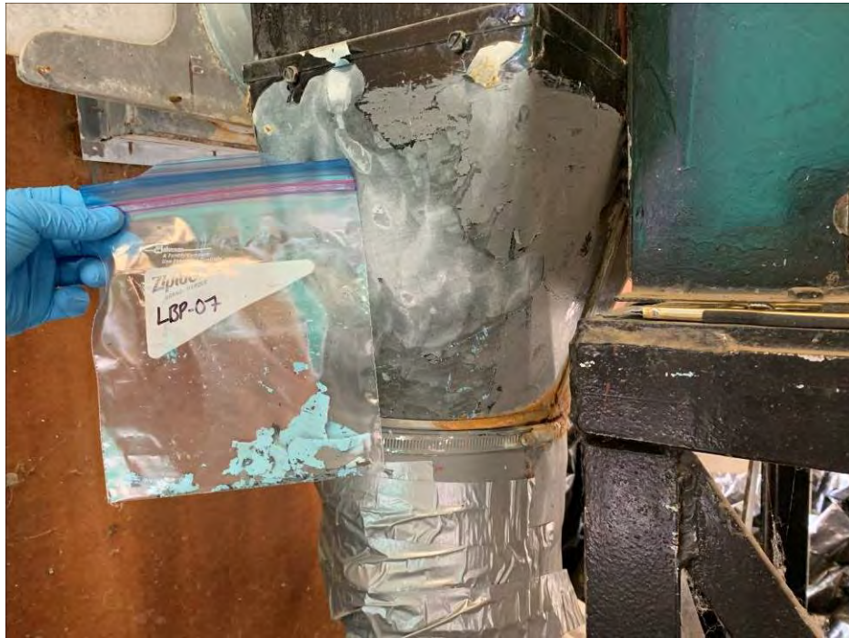
Photo 11: General view of the paint chip sample LBP-07 location on the piping for the blower near the northeast corner of the main floor. (April 27, 2021)
