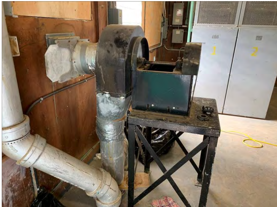
Photo 12: General view of the blower and associated stand on the northeast corner of the main floor. (April 27, 2021)
