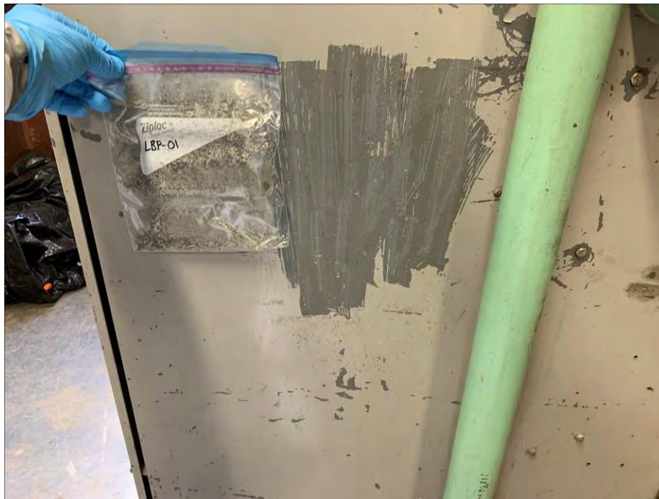
Photo 2: General view of paint chip sample LBP-01 location on electrical components on the main floor. (April 27, 2021)
