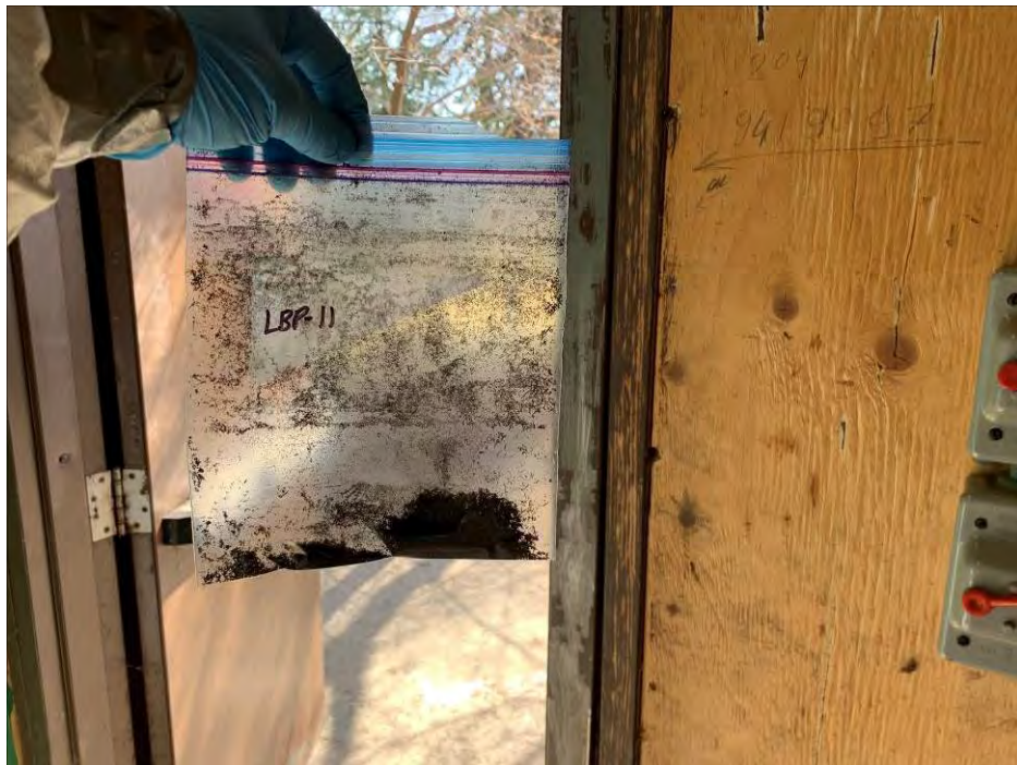
Photo 19: General view of paint chip sample LBP-11 location on the door frame at the northeast corner of the main floor. (April 27, 2021)
