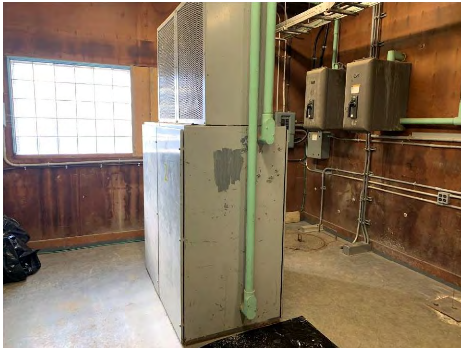
Photo 1: General view of electrical components on the main floor. (April 27, 2021)
