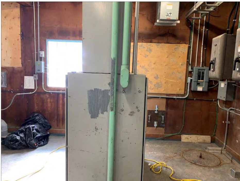
Photo 14: General view of the conduit connecting electrical components on the main floor. (April 27, 2021)
