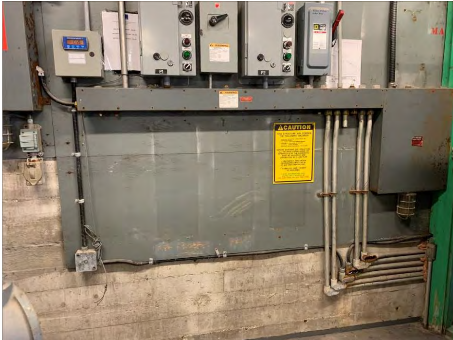
Photo 5: General view of the plywood backing board for the electrical panel on the north wall of the main floor. (April 27, 2021)
