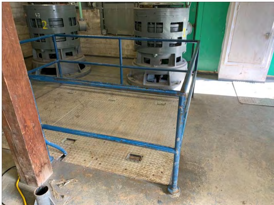
Photo 16: General view of the guard rail near the center of the main floor. (April 27, 2021)
