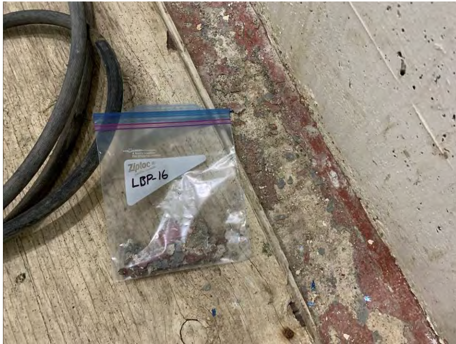
Photo 27: General view of the paint chip sample LBP-16 location on the floor in the motor room. (April 27, 2021)
