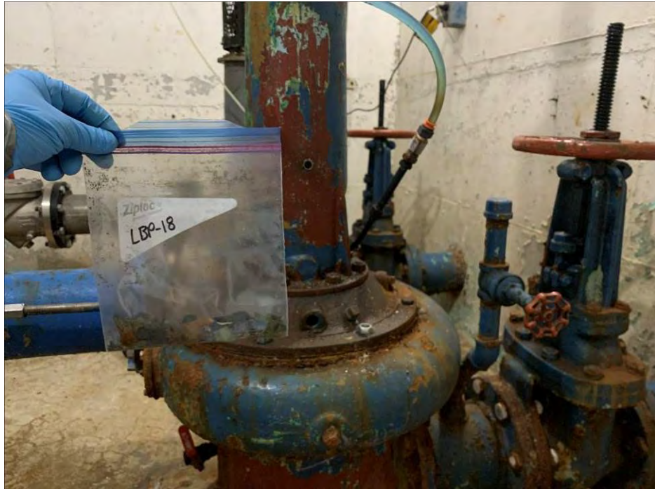
Photo 31: General view of the paint chip sample location LBP-18 location on a pump in the pump chamber. (April 27, 2021)
