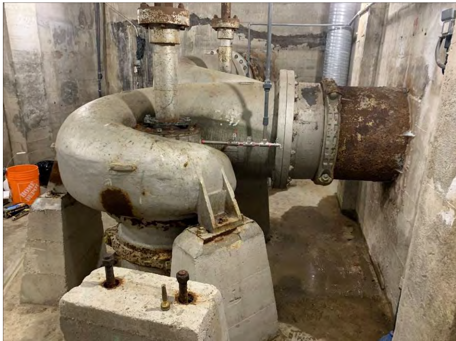
Photo 22: General view of the centrifugal pump P-46 in the dry well. (April 27, 2021)
