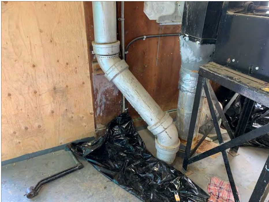
Photo 10: General view of the blower and associated piping near the northeast corner of the main floor. (April 27, 2021)
